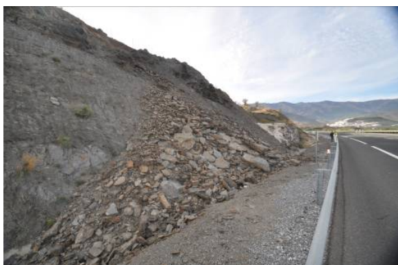
Fig. 6 Landslide in a road embankment in the kilometric point 339 belonging to the A92 dual carriageway, Spain.
