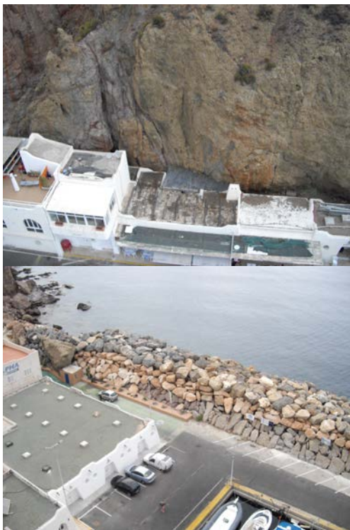
Fig. 23 San José Port. Two points of view taken from a fix helix UAV for stability talus control.
