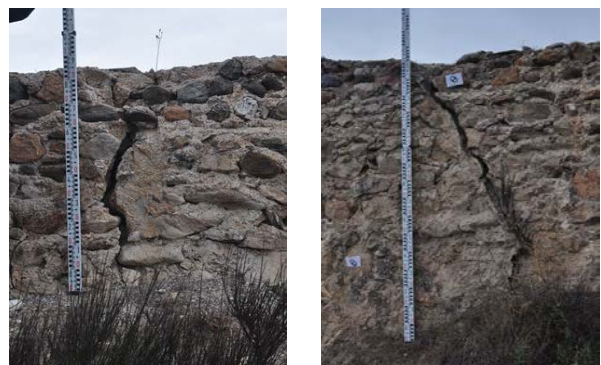
Fig. 16 Detected splits crossin both faces of the wall.
